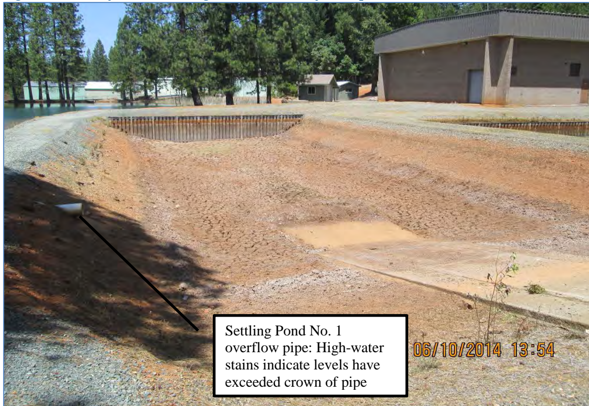
Figure 7. Photo of FWTP Settling Pond No. 1 Overflow Pipe
